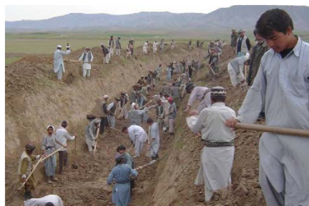
ALP/N organized and financed cash-for-work activity in Northeast Afghanistan. About 19,700 workers received an average of US$50 per person and accounted for roughly 197,000 days of labor. The activity accounted for a major renovation of the irrigation network, providing farmers with additional water capacity. PHOTO: PADCO-AECOM
